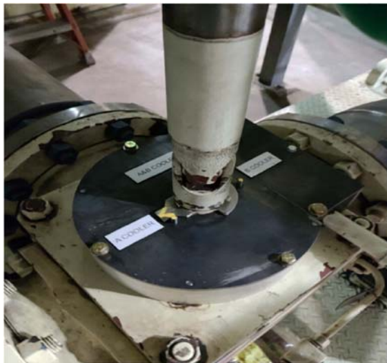
Figure 14. 6-way valve position indicator as modified.
